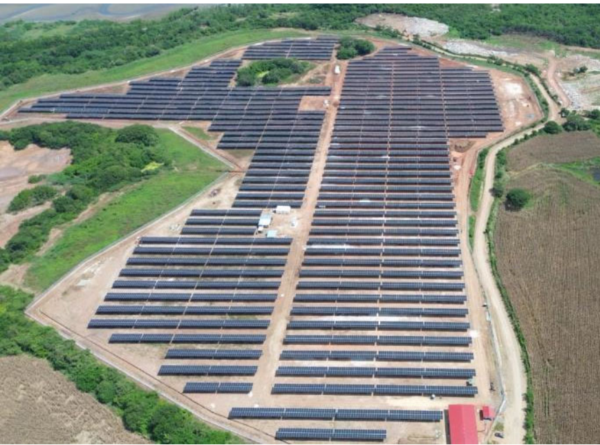
Located in Los Santos Planta conected to the grid Generating 100%
