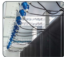
Wall Socket Minimal Cooling
