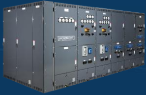
AMC SWITCHGEAR & TRANSFER SWITCHES
