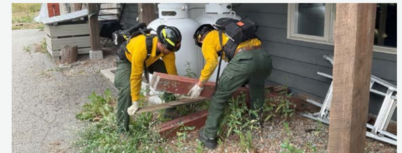
Wildfire Defense Services personnel relocating combustibles to reduce potential sources of ignition adjacent to the primary structure.
