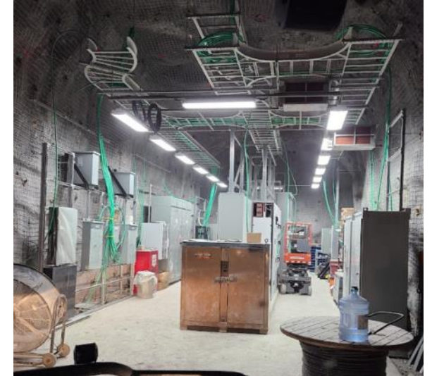
ERU 9 Electrical Room
