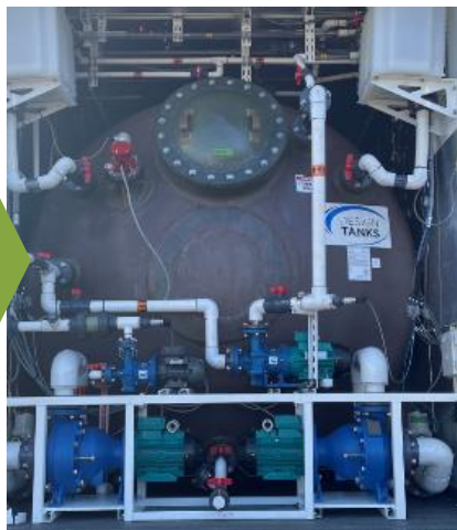
Electrical wiring and component reduction
