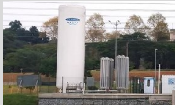
Municipal SDOX system for water treatment
