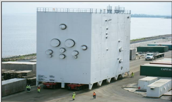
IPSMR® liquefaction process and cold boxes for Phase 2 Woodside Louisiana LNG
