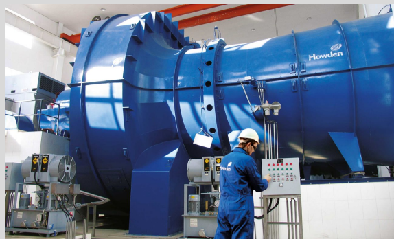
Fans for mining customer
