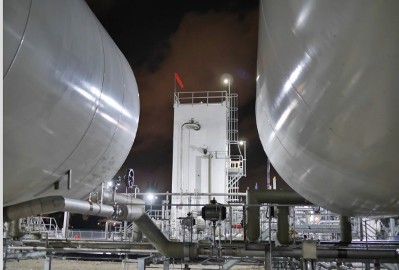
IPSMR® liquefaction process and cold boxes for Phase 1 Woodside Louisiana LNG
