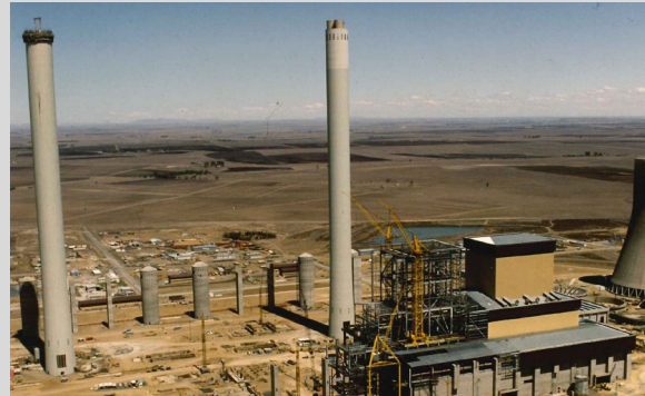
African Power Utility AH recovery project installation
